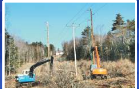
10.1 MILES - 69 kV TRANSMISSION LINE
