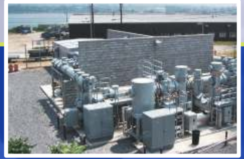
GAS INSULATED SUBSTATION
