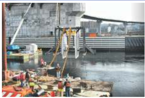
BRIDGE CONTROL SYSTEMS SUBMARINE / CATENARY
