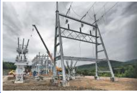
EPC PROJECT - 34.5 / 115 kV WIND FARM COLLECTOR SUBSTATION
