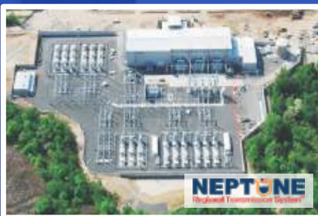
NEPTUNE CONVERTER STATION
