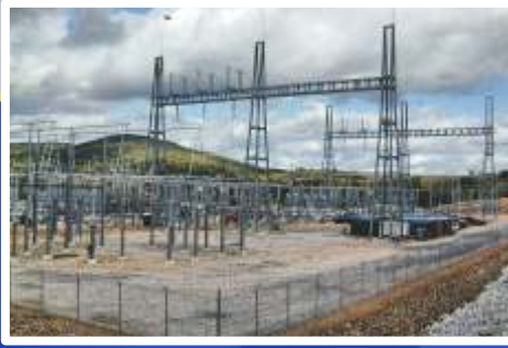
9 ACRES - 345 / 115 kV SUBSTATION
