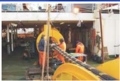
65 MILES - SUBSEA HVDC CABLE
