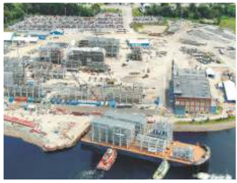
Offshore Wind Facility
